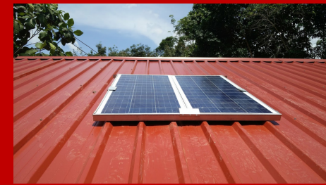
Figure 4: Solar panels attached to the roof
