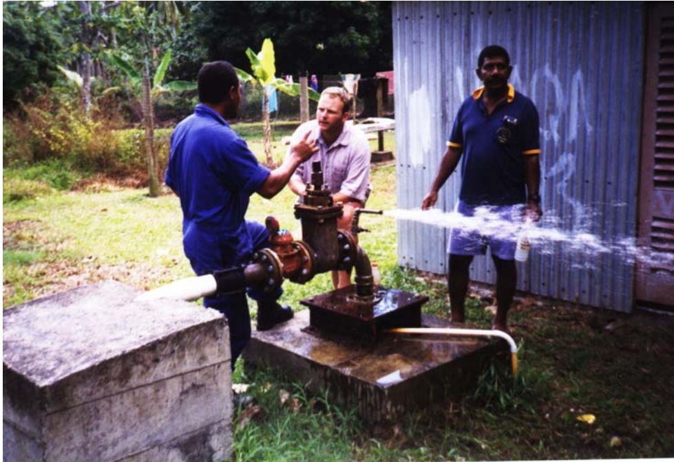
A pump test being carried out by MRD and ourselves at the Daliconi site.
