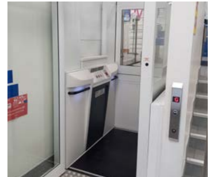
AN ACCESSIBLE LIFT, THIS ONE IS IN THE ETHOS BUILDING
